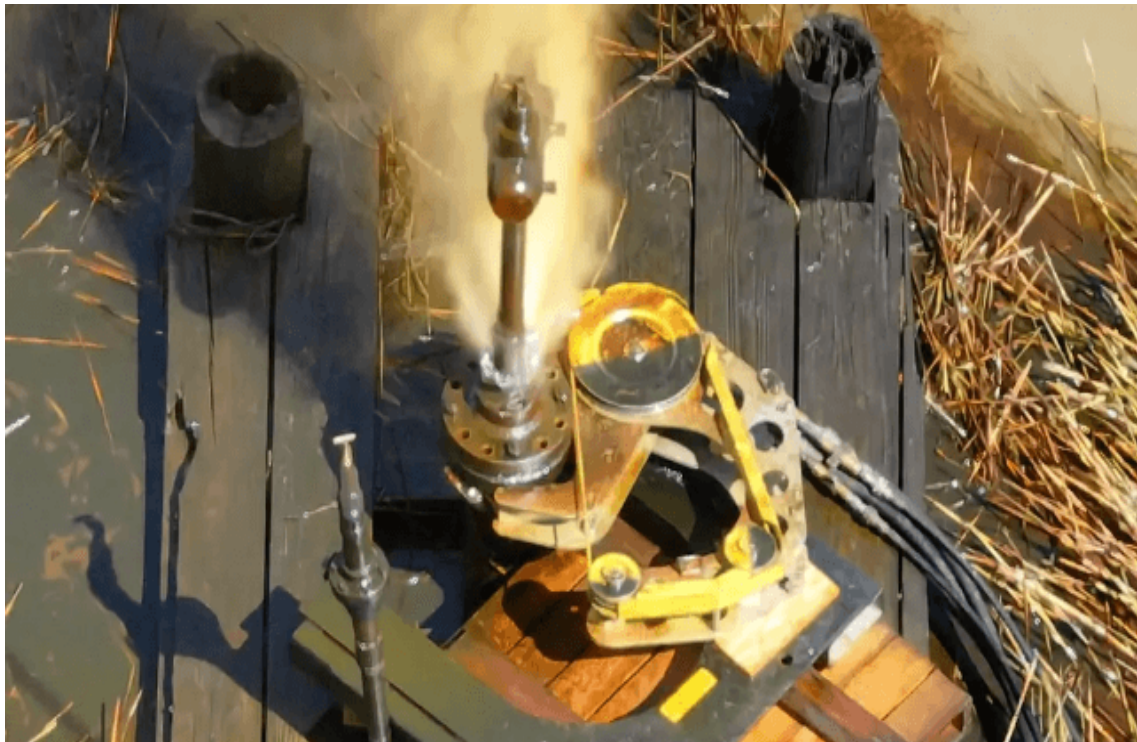
Contractors prepare to cut off the leaking wellhead at the flange (USCG) Source: US Coast Guard
