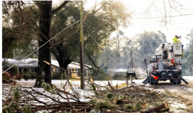
Vegetation damage has contributed to longer restoration times in some areas Source: Entergy
